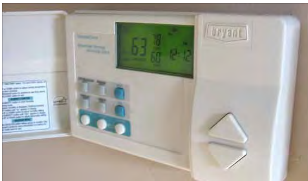
Many types and designs of electronic setback thermostats are available. The model above is for a heat pump.
