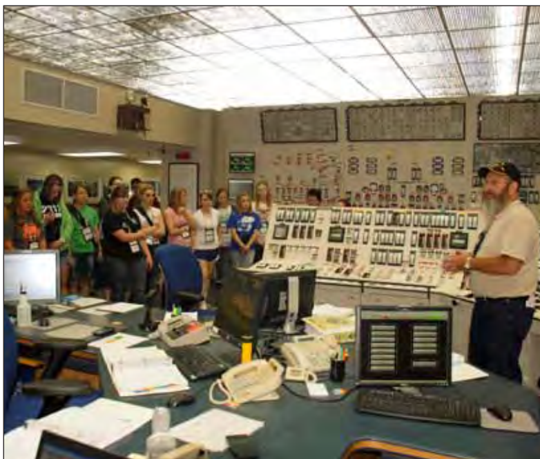
A mockup of the Wolf Creek Nuclear Generating Station's control room, used for training, was one of the places visited by the Government In Action Youth Tour students this summer.
